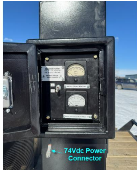
Figure 2: 74Vdc Connection / Instrumentation Compartment
